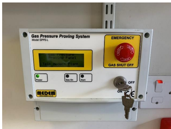
Figure 3: Gas pressure proving systems (propane) in the off position.
