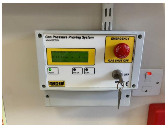
Figure 4: Gas pressure proving systems (propane) in the on position.
